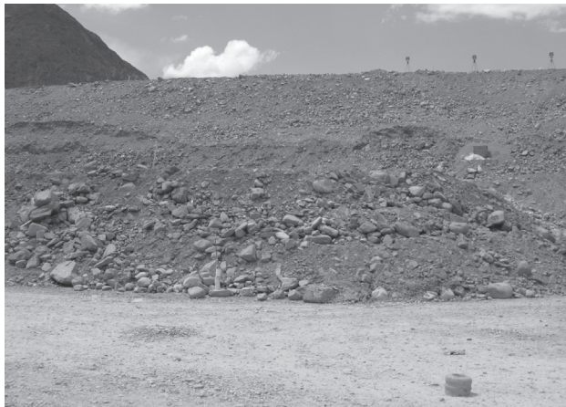
Figure 3 - Caracoles dam under construction (2007). San Juan, Argentina. Detail of the gravel fill.
