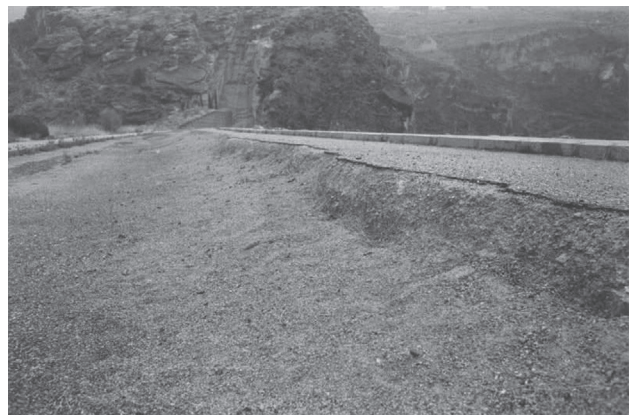
Figure 11 - Collapse settlements of rockfill in Martín Gonzalo dam, Córdoba, Spain.
